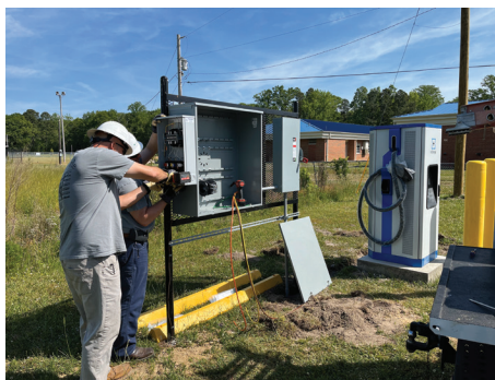
Manager of Technical Services Travis Riddick and Engineering Technician II Timothy Meads work on the current transformer and meter for the electric school bus charging station at Camden Middle School.
